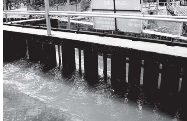
Fig. 18.4 Grit and sand removal tank
